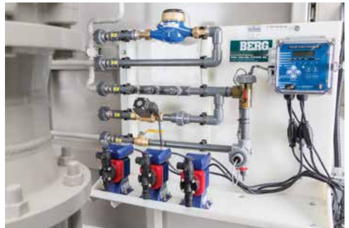
Chemical Treatment System provides proportional chemical feed and bleed-off to make-up.
