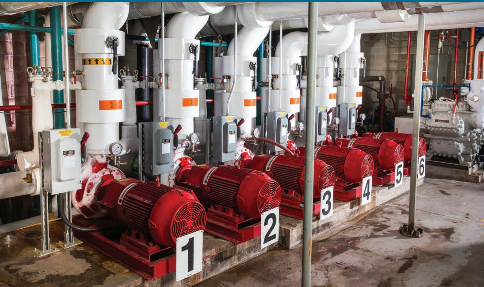
Max efficiency and control - glycol pumps with variable frequency drives each feed a specific rink
