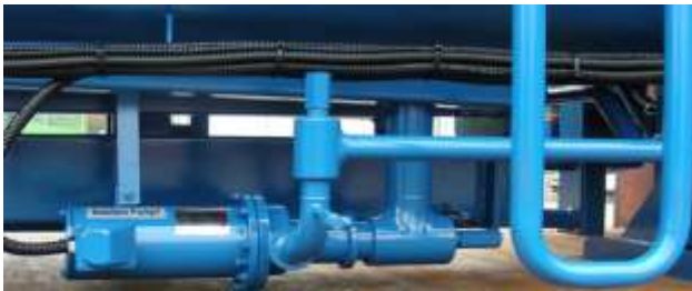
Canned type pump & Isolating Valves (Angle valves)
