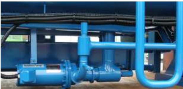
Canned type pump & Isolating Valves (Angle valves)
