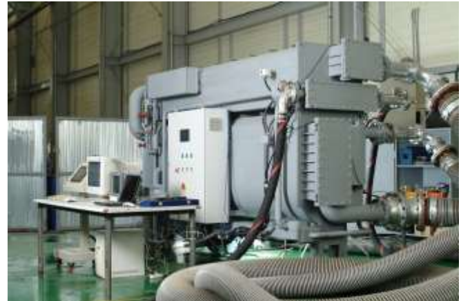
Test of Absorption Chiller
