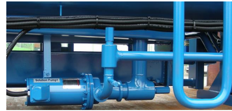
Canned type pump & Isolating Valves (Angle valves)
